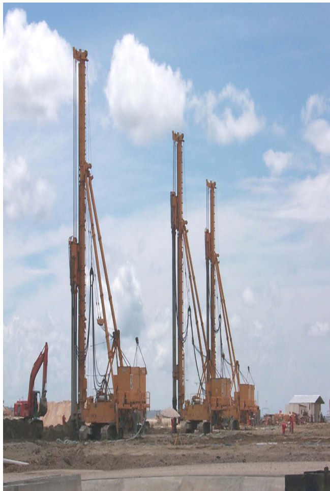
Up to three soil mixing rigs worked two shifts to complete the project on time
