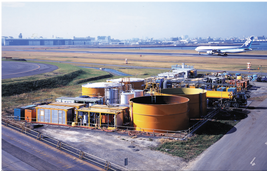
MaxPerm grout plant for liquefaction prevention work at Tokyo International Airport (Haneda)
